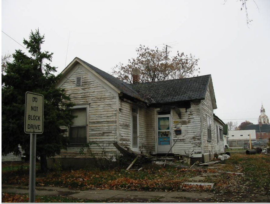
Dilapidated, Vacant House
