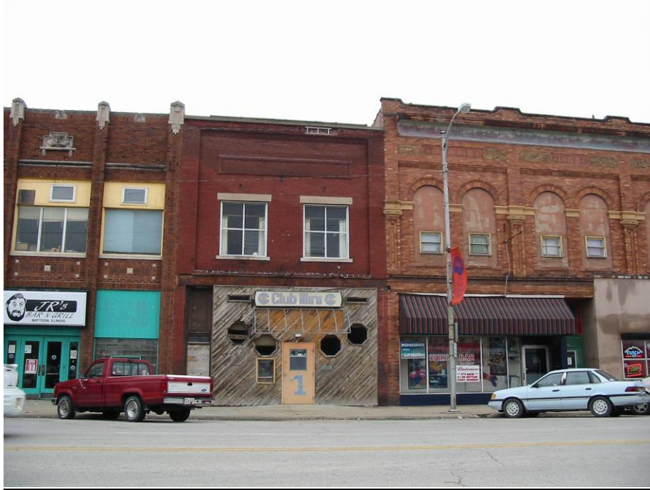
Vacant, Obsolescent, Deteriorated Commercial/Residential
